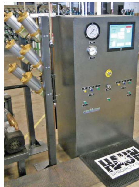
Automated oxygen filling system
