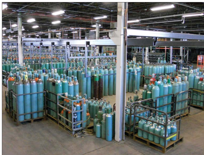
New Haun Specialty Gases plant boasts a 120 x 20-foot fill island with traversing manifolds.
